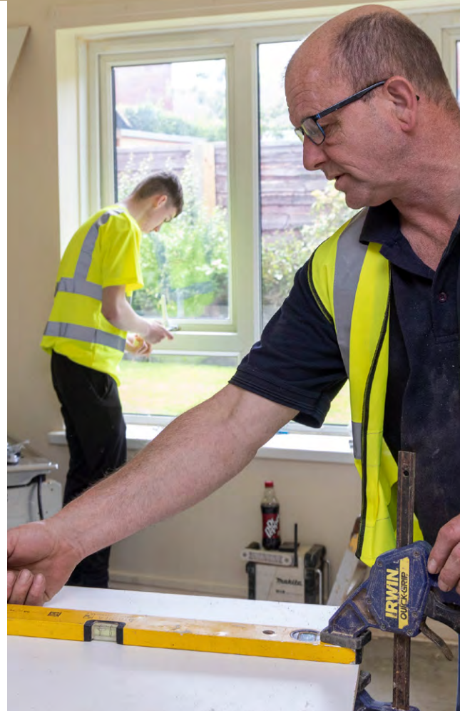
Stockport's B4Box give paid, on-the-job retrofit training to marginalised young people – delivering skills and support into work. The organisation won an Ashden Award in 2022.
